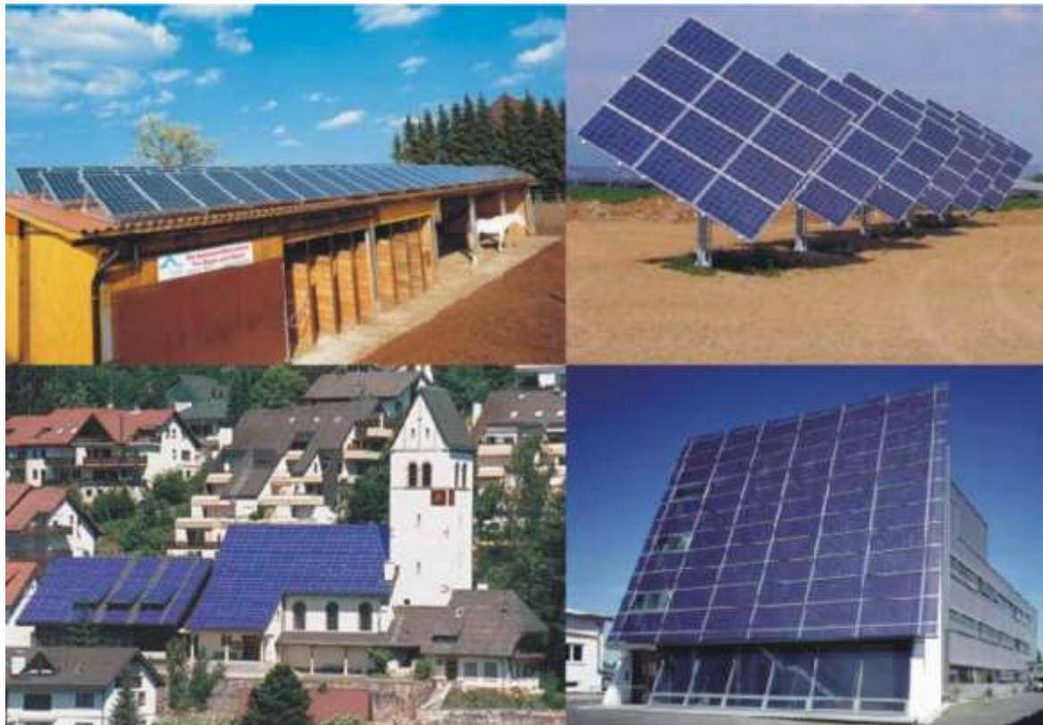
Figure 6. Ground-mounted and building-integrated photovoltaic arrays (J. Beseničara et al, 2008).
